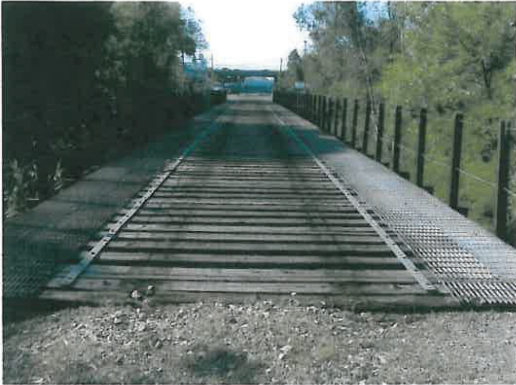
Figure 3: View of wood deck of former railroad trestle over Los Gatos Creek
