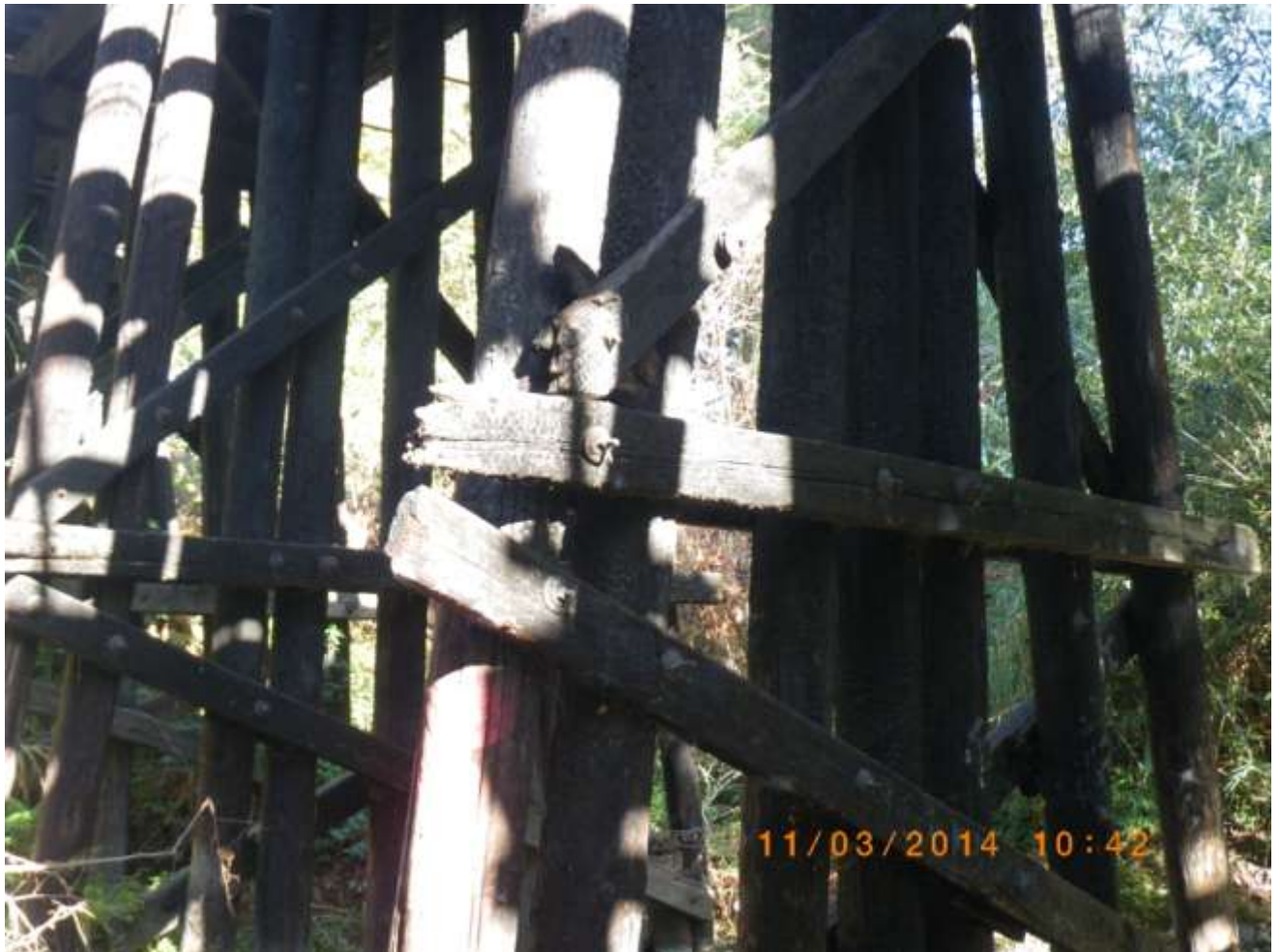
Photo #8. Weathered and splintering pilings on railroad trestle in disrepair. 3 November 2014
