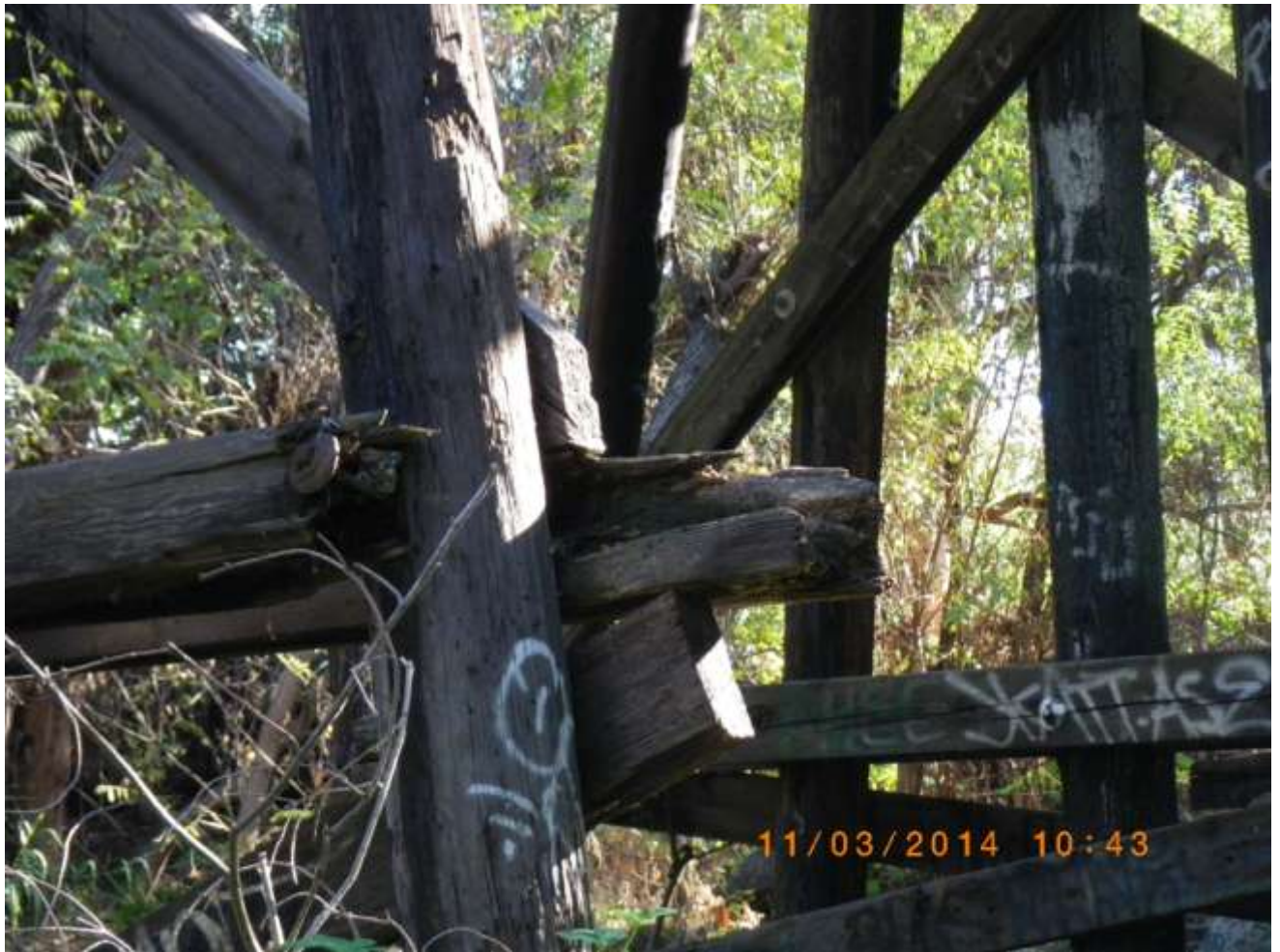
Photo #9. Weathered and splintering pilings on railroad trestle in disrepair. 3 November 2014
