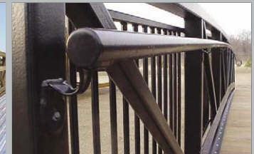
Vertical Picket/Pipe Handrail
