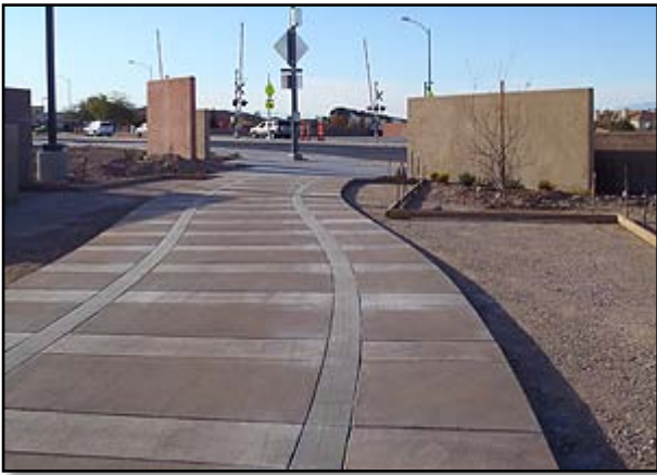
Figure 1: Concrete Stain Example
