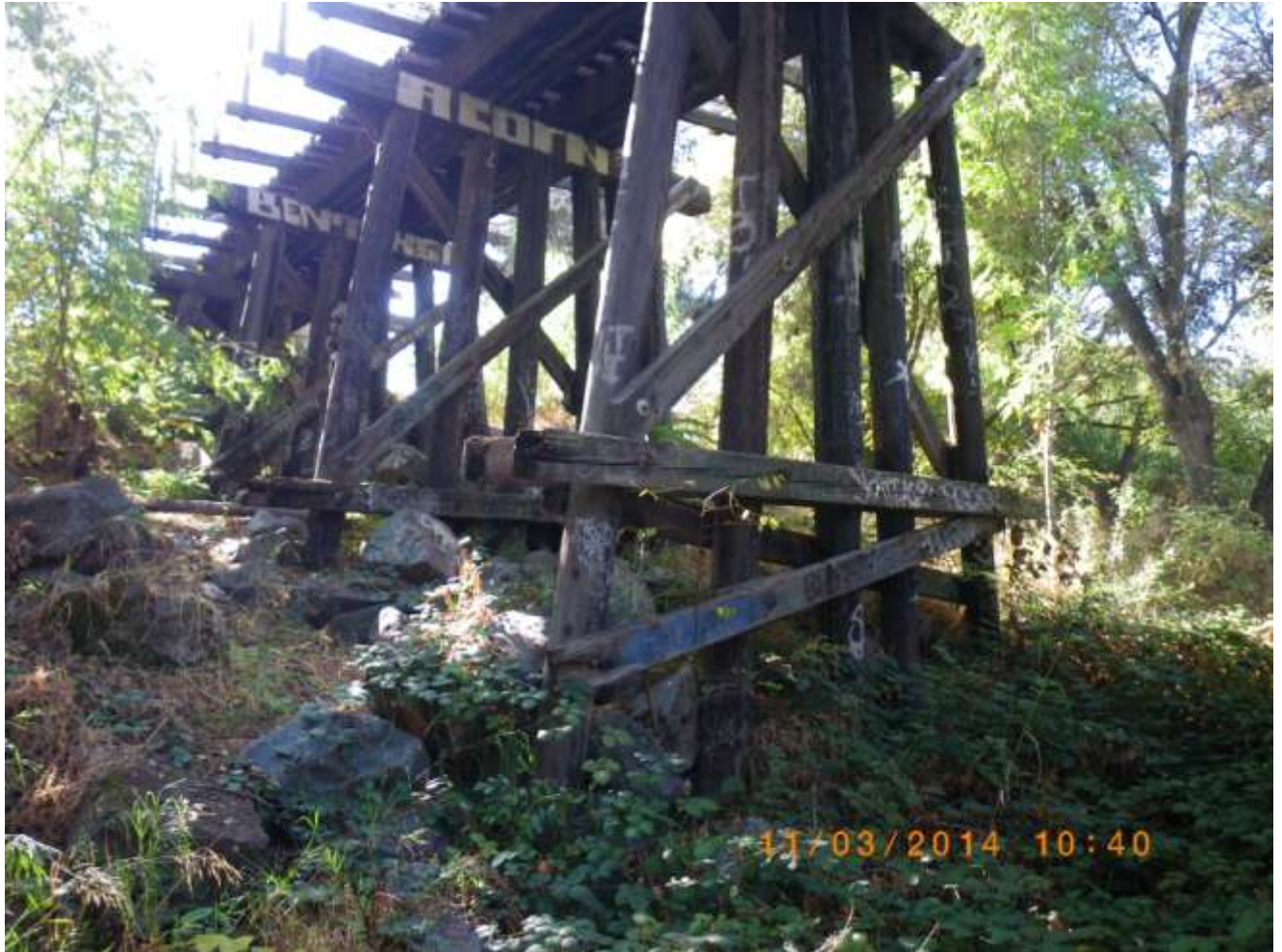
Photo #14. Riprap under railroad trestle (weathered pilings), south side. 3 November 2014
