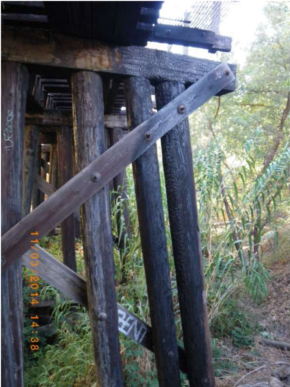
Photo #10. Charred pilings on railroad trestle, north side. 3 November 2014
