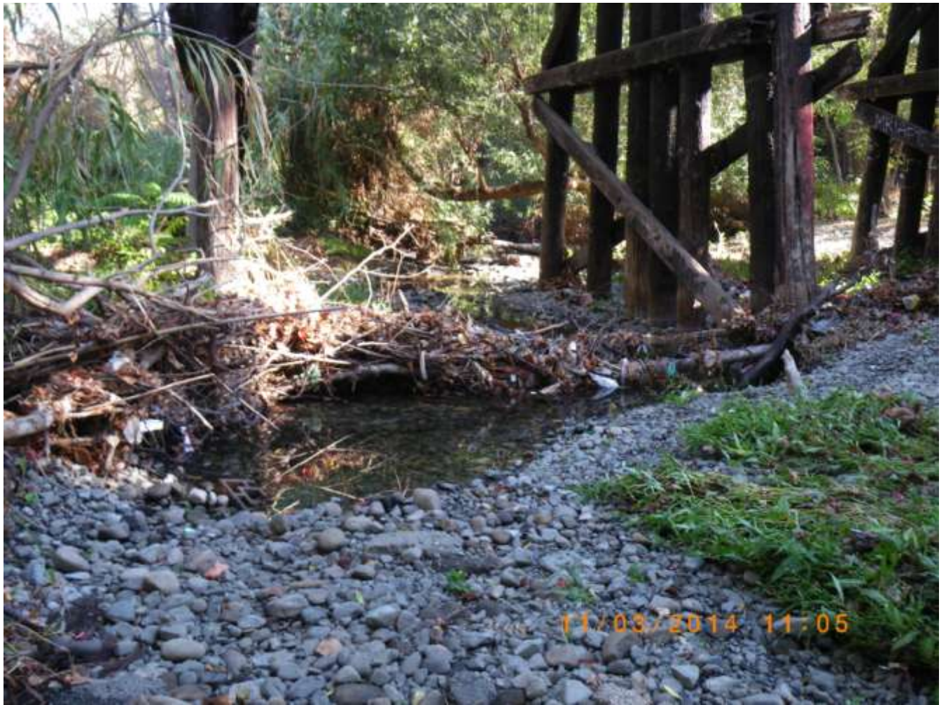
Photo #11. Woody debris collected on railroad trestle pier. 3 November 2014
